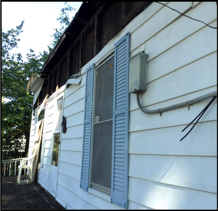
Front face porch missing roof of 319 Monroe St
