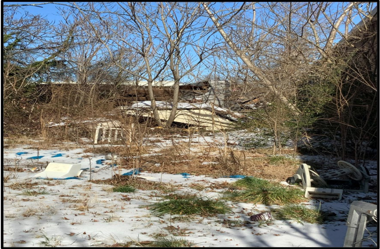
Rear addition and collapsed accessory structure
