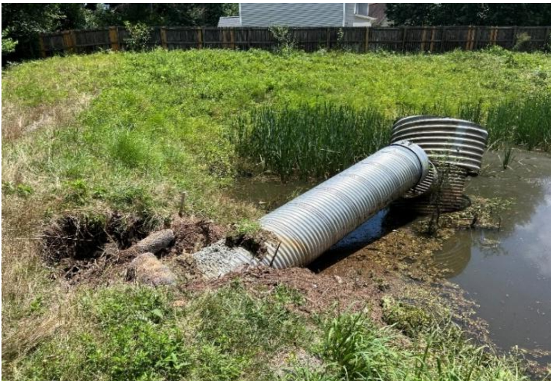
Figure 6-1. SCM outlet and dam failure
