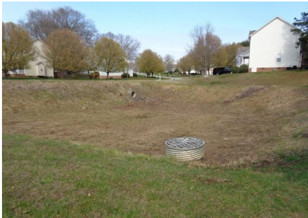
Figure 5-5. Dry detention pond
