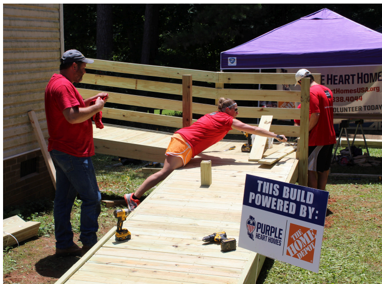
ADA ramp installation at a Veteran's home, sponsored by The Home Depot
