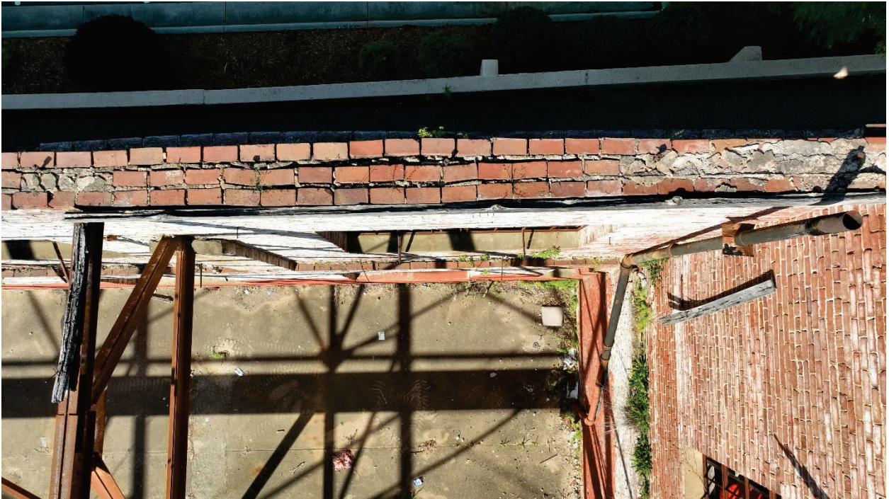
Photograph 3: Loose brick along the top of the west wall.
