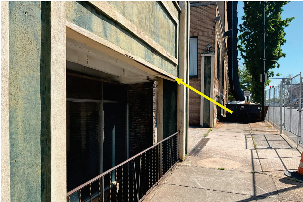
Photograph 11: Deterioration in the cosmetic surface of the porch area.
