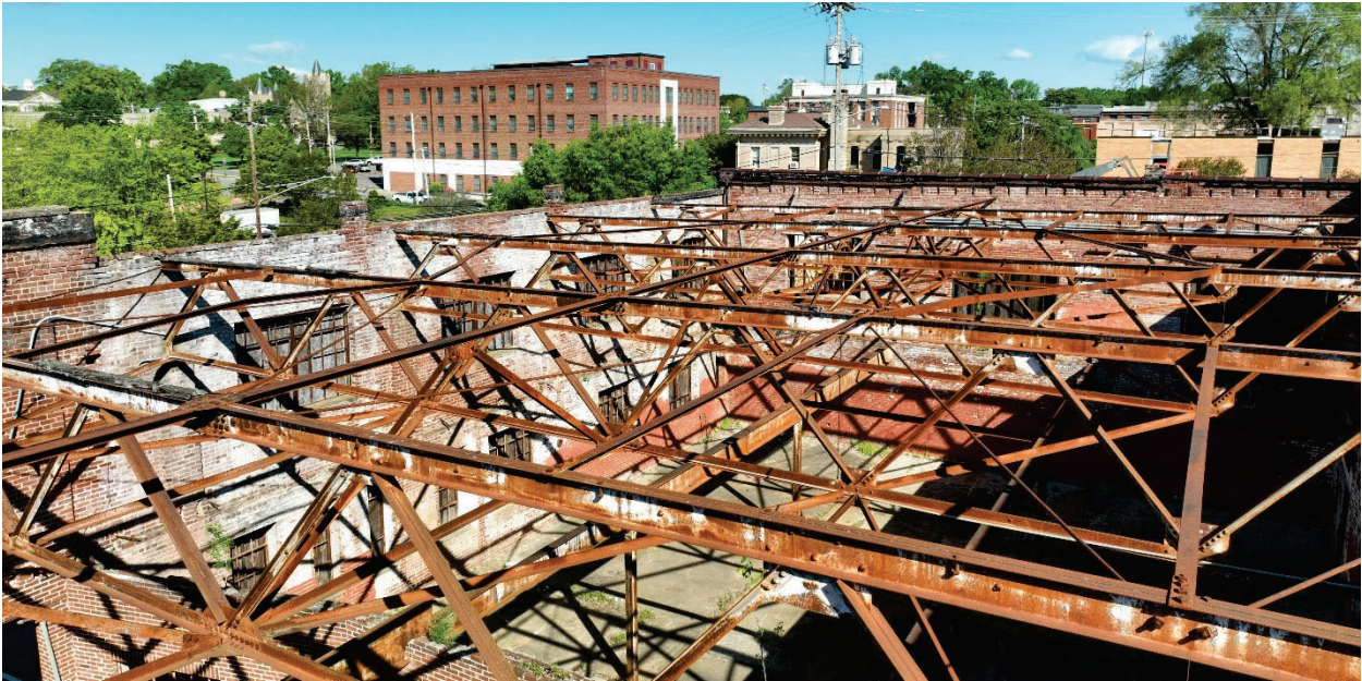
Photograph 1: No roof framing is present.
