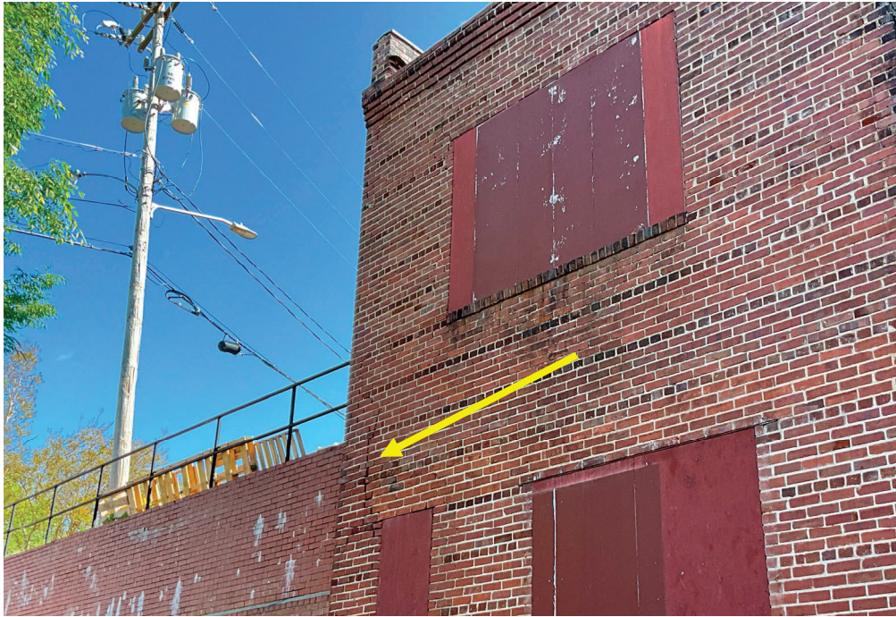
Photograph 7: Cracks at the northwest corner of the wall.
