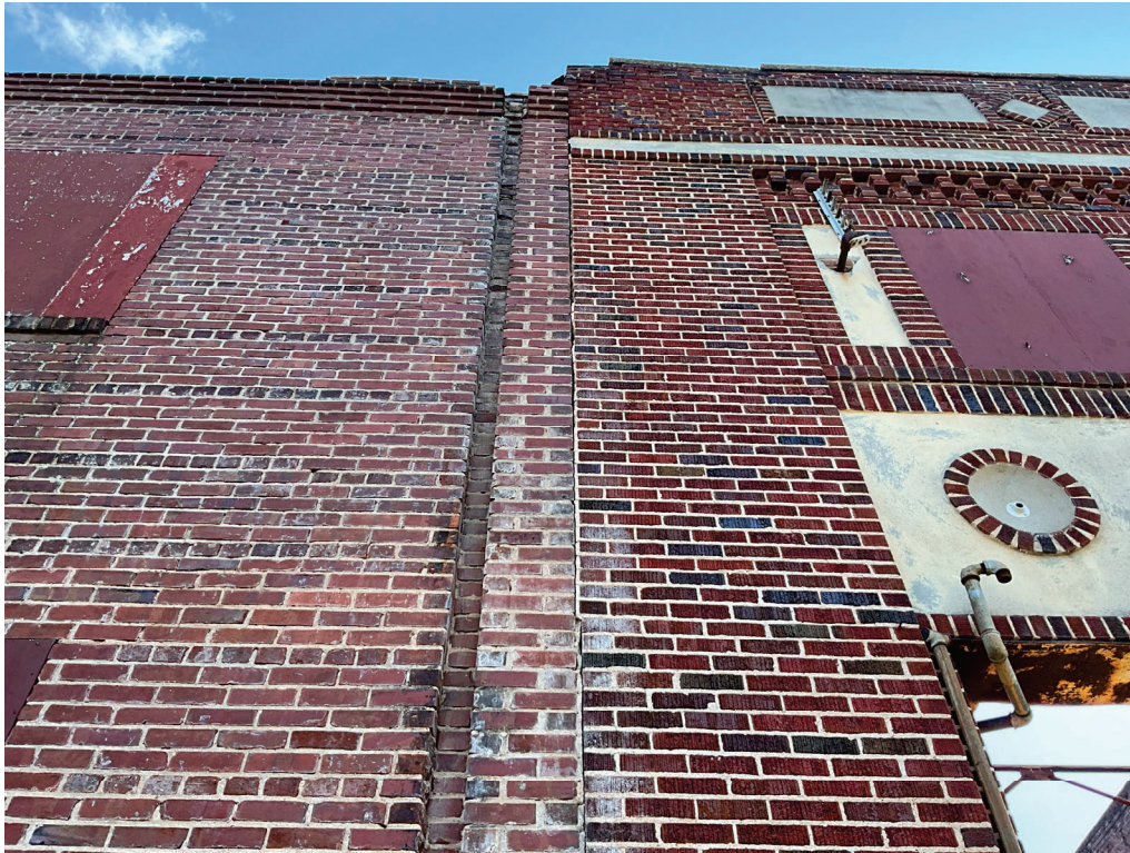
Photograph 9: Same cracked wall area as Photograph 8, as seen from the outside.
