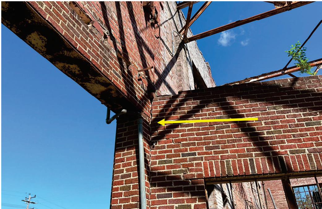
Photograph 8: Cracks at the wall intersection on the west side.
